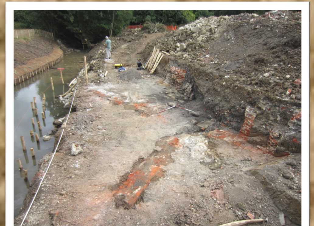
Brick walls of the incorporating mill in the left hand bank of the Hogsmill river cut through by the environmental works in 2013
