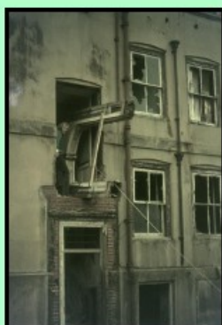
Above- A door frame being rescued from The Shubbery prior to demolition
